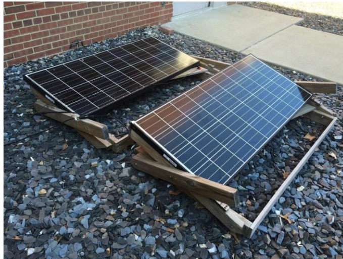
Figure 1.1: Solar panel configuration
