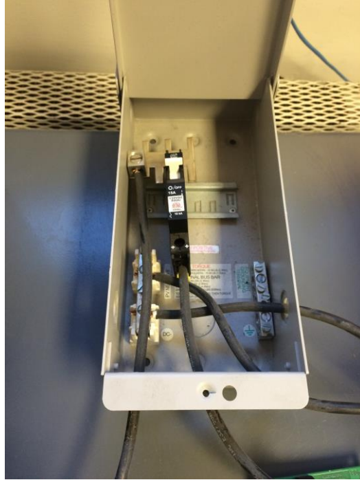
Figure 1.3: Solar panel combiner
